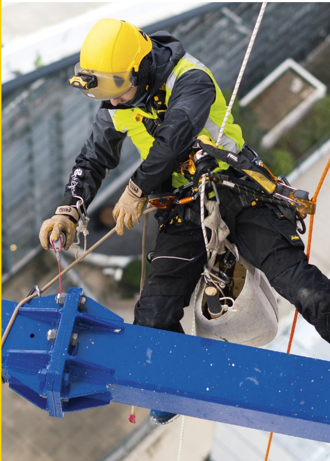
Repositioning the braces of a tower crane, France © 2019 - Petzl Distribution - Vuedici.org - Integral - Bateg - Tour Trinity - Cro&Co Architecture
