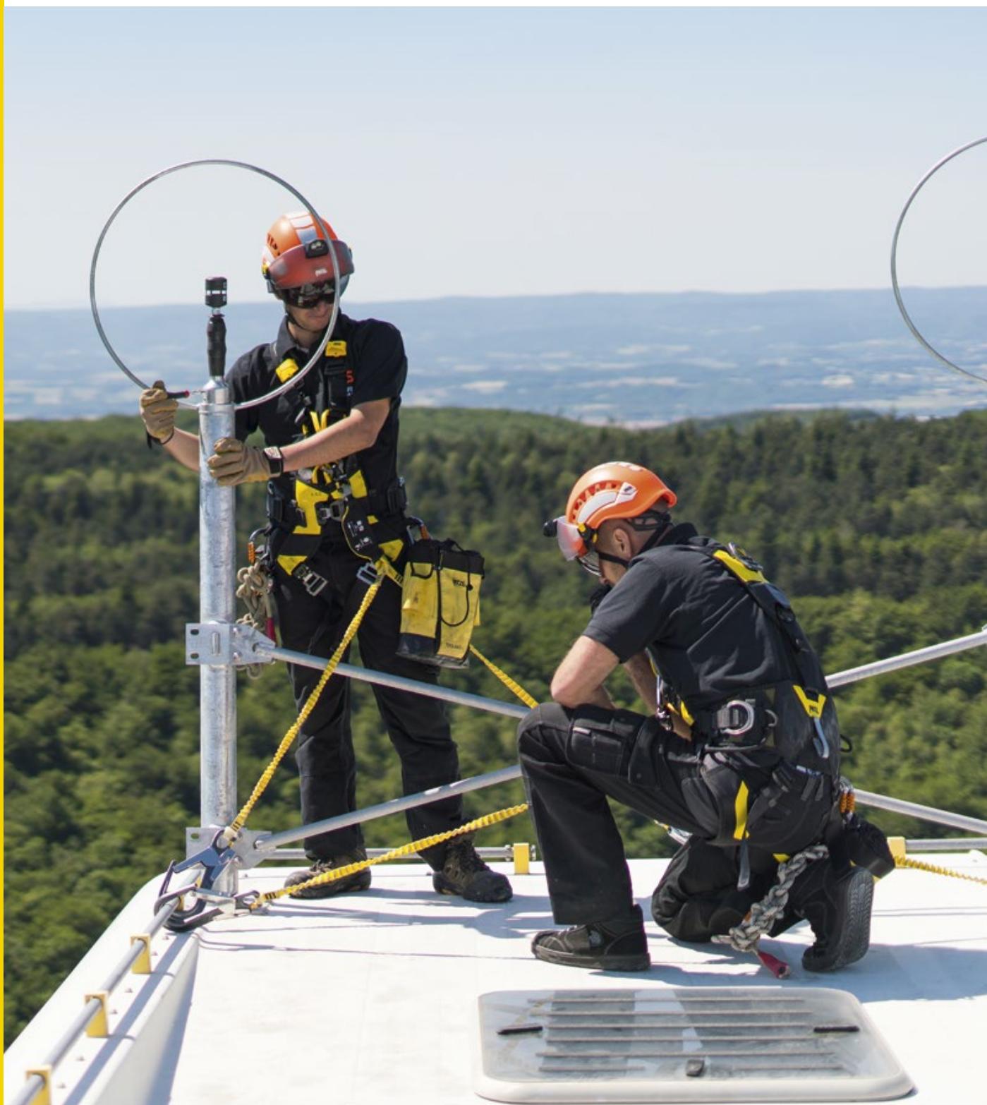
Maintenance operations of wind turbines, France © 2019 - Petzl Distribution - Vuedici.org - RES - Parc éolien de Marsanne
